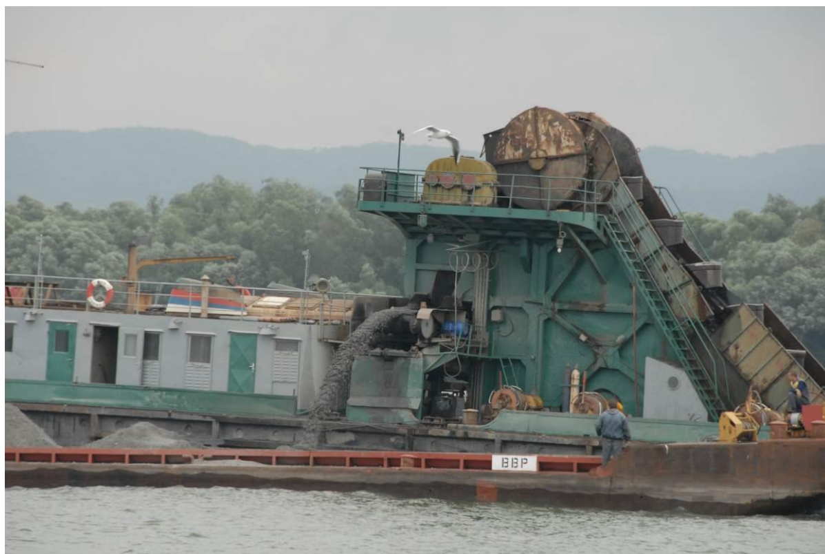
Figure 7: Particular dredging activities exceeding regular maintenance dredging affecting > 500 m reaches should be recorded (photo credit: Wolfgang Kraier).
