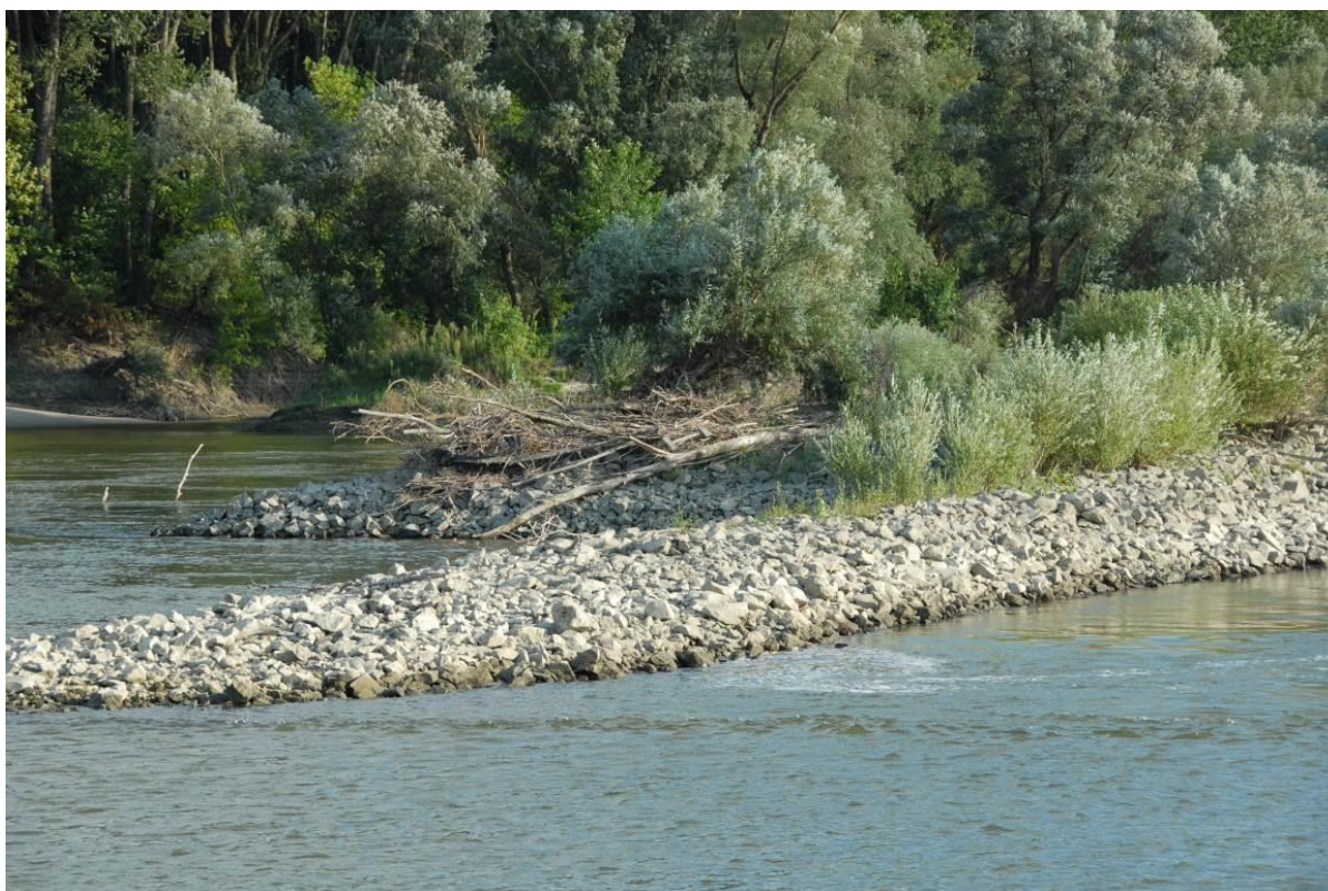
Figure 8: New established or enlarged groynes influencing flow conditions > 500 m reaches (also groin fields, guiding walls or new chevrons should be recorded (photo credit: Wolfgang Kraier).
